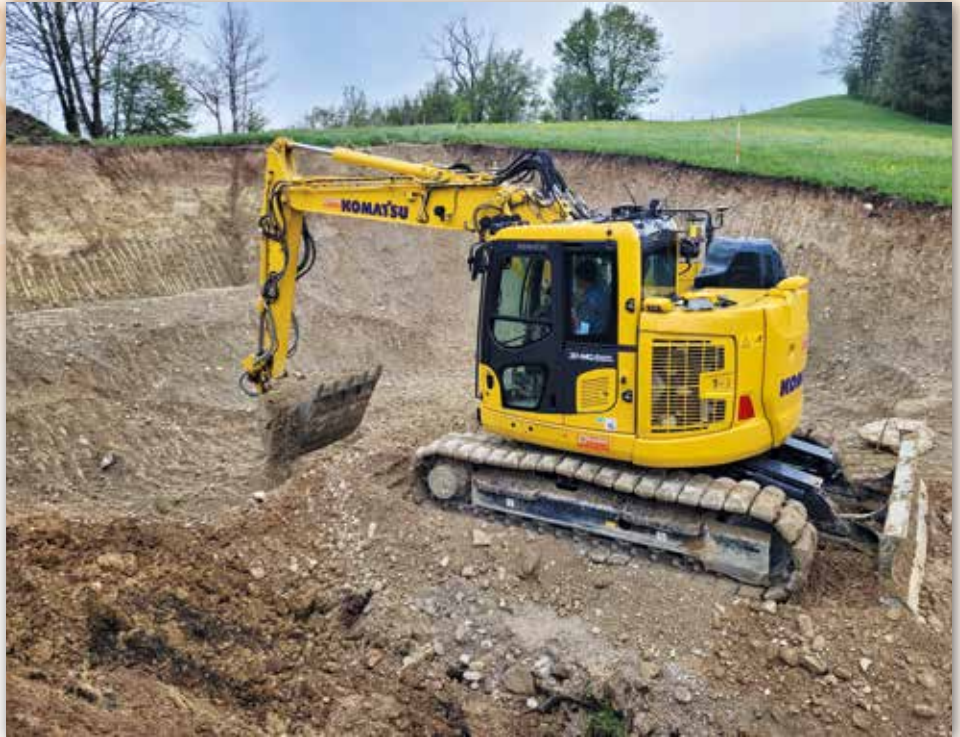
Together with Smart Construction 3D Machine Guidance, the Komatsu PC138US-11 is perfect for Froschauer GmbH's area of application.
